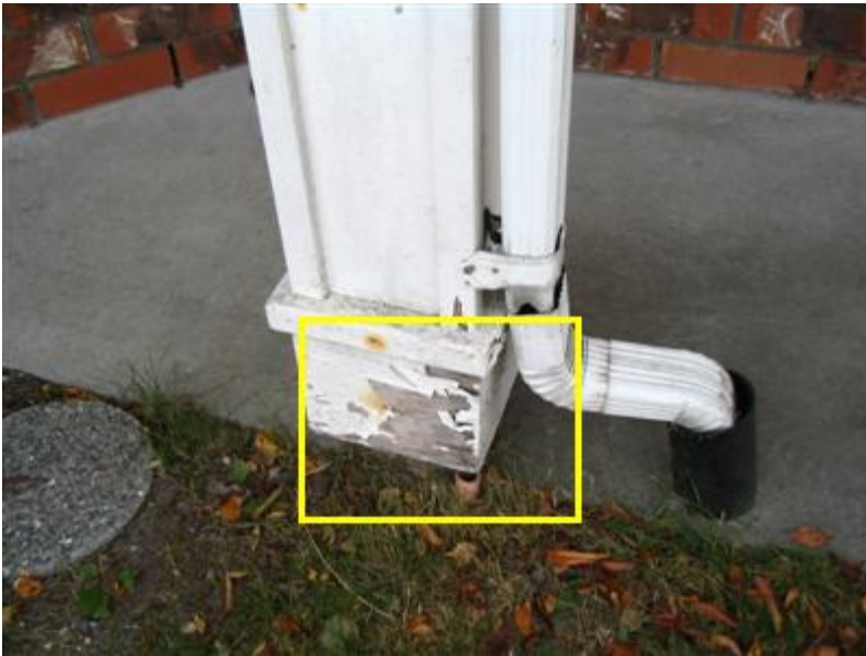
2.1 Picture 1 Paint repairs required
