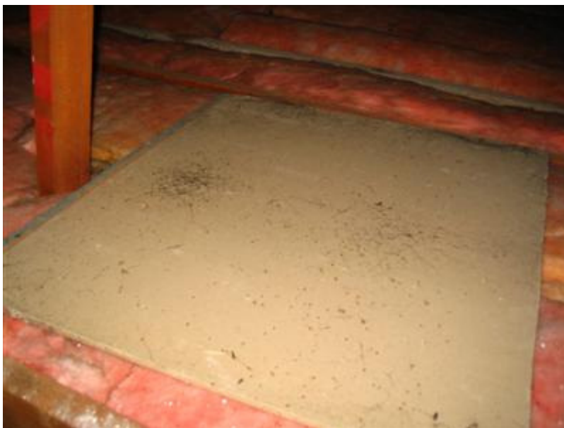
9.0 Picture 1 Attic access cover
