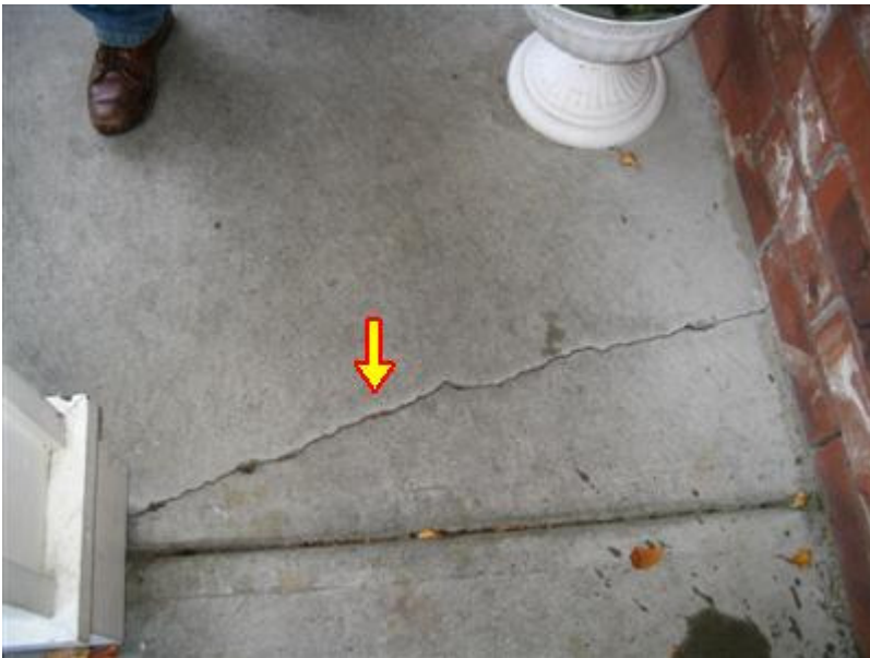
2.9 Picture 1 Cracked walkways
