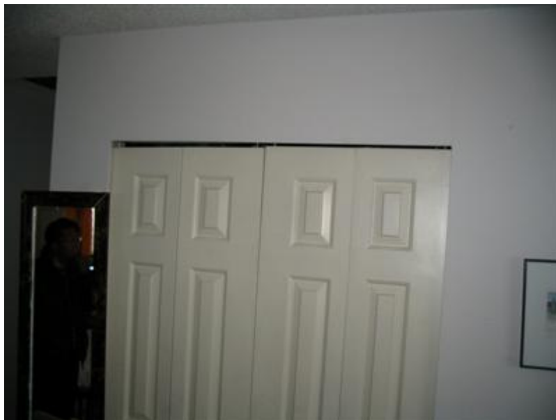
5.1 Picture 1 Door jamb not level
