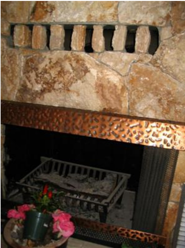
8.0 Picture 1 Chimney Cleaning required
