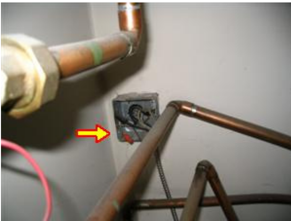
8.1 Picture 1 Wire disconnected in boiler closet
