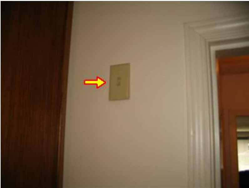
8.2 Picture 1 Boiler switch not functioning
