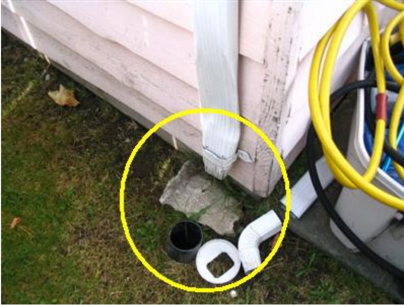
2.5 Picture 1 Damaged/disconencted drain
