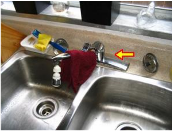
6.10 Picture 1 Loose tap
