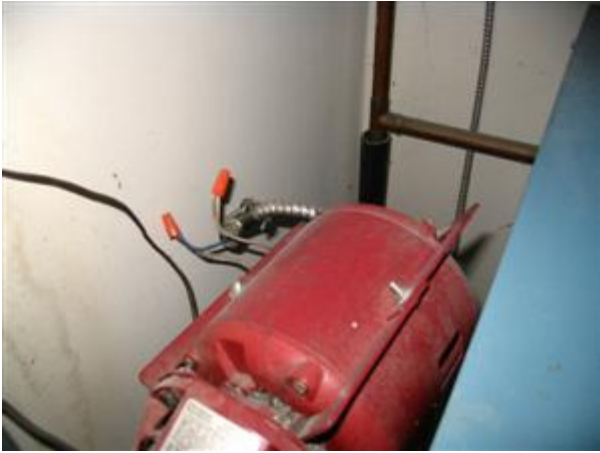
7.4 Picture 1 Loose wiring
