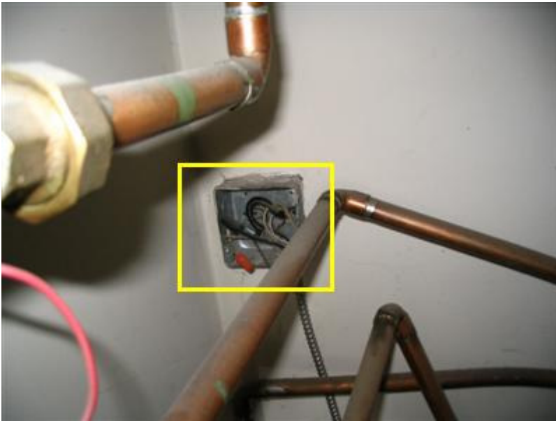
7.10 Picture 1 Missing cover plate
