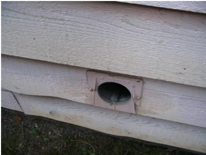
9.3 Picture 2 Dryer duct outlet
