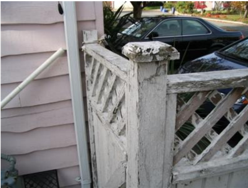
2.8 Picture 1 Weathered fence
