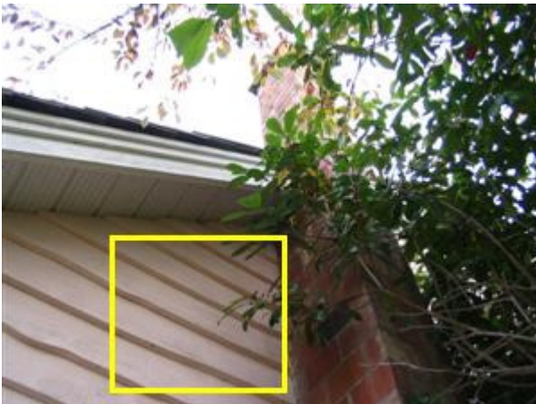
2.1 Picture 2 Paint repairs required
