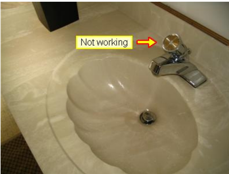
6.9 Picture 2 Faulty tap
