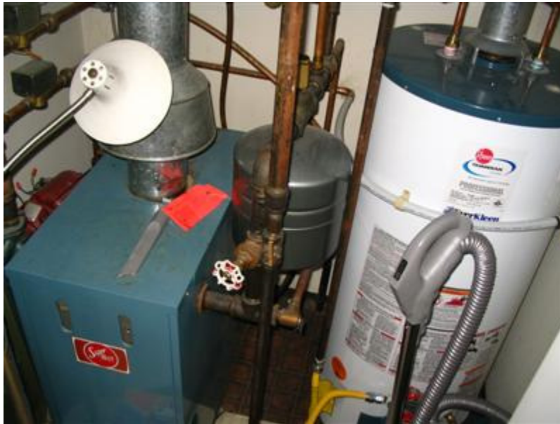
Boiler and water heater
