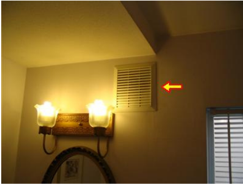
9.3 Picture 1 Fan not working
